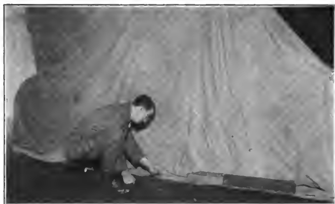
Fig. 1.—Care should be taken to see that the cover is either held to the ground or tacked thereto
